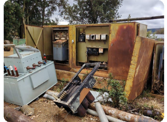
Decommissioned transformers, switchgear and cabling on site at Umvoti Municipality.
