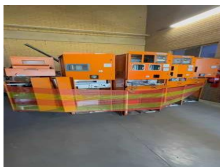
Industrial Electrical Switchgear / Merlin Gerin Substations (Lots 292, 294, 313)
