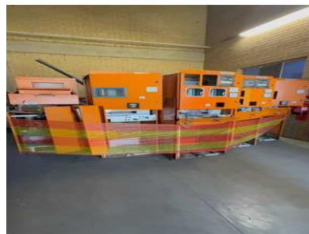
Industrial Orange Electrical Switchgear Units
